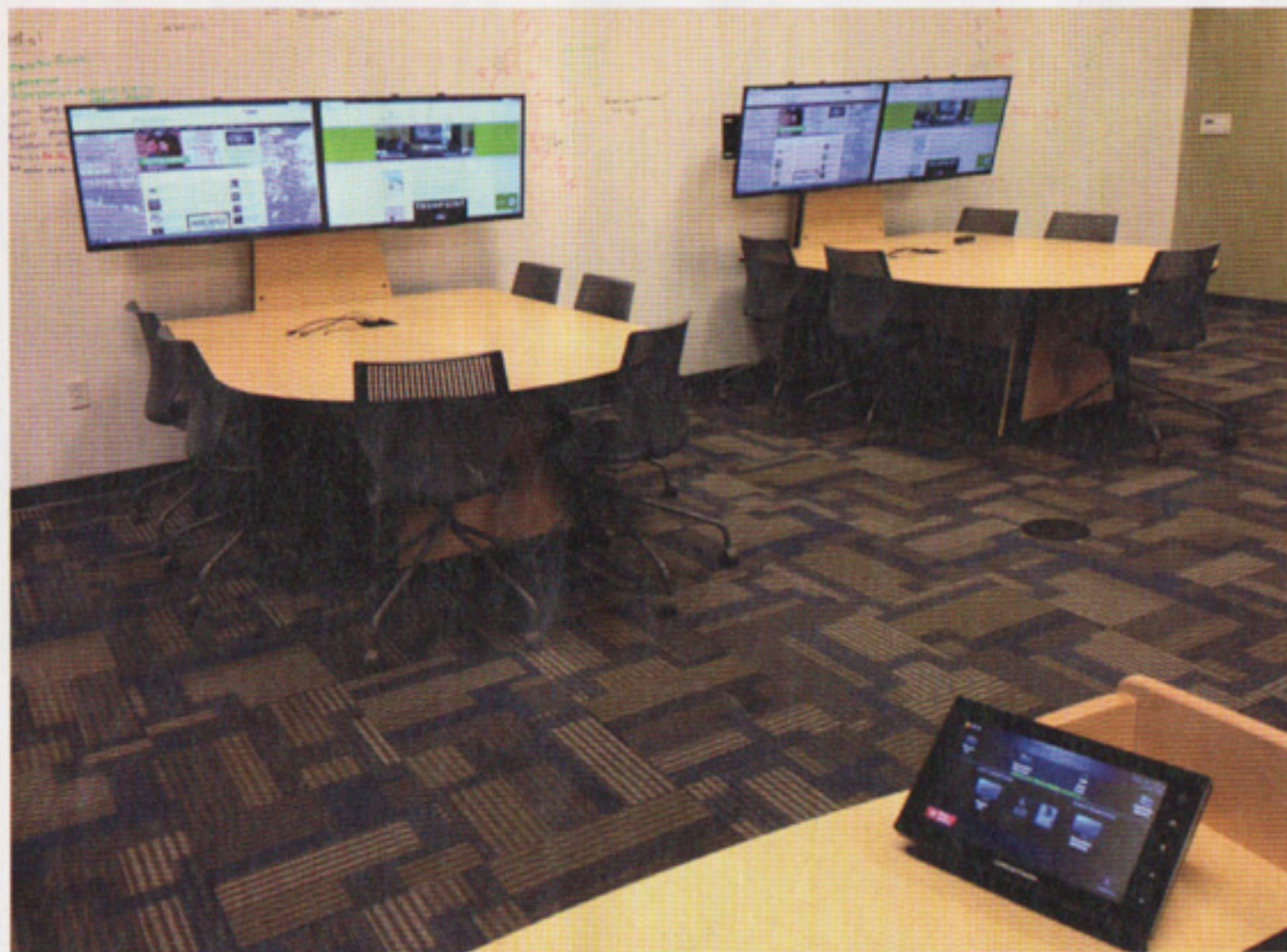
Marian University in Indiana is outfitted with the latest control, video, and audio technology. This collaborative space is also equipped for multiple uses.
